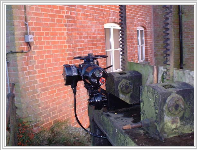
A closer view of the penstock sluice gate with a Rotork actuator attached
