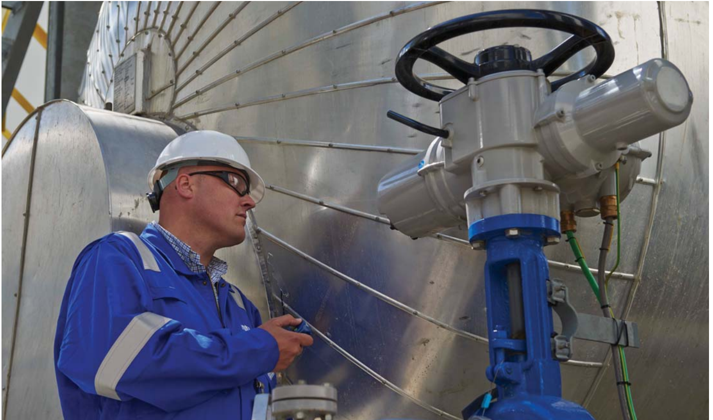
Fig 1 - The IQ actuator provides a 'window into the conditions' at the valve.
