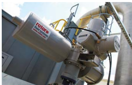
Rotork Skilmatic electro-hydraulic failsafe actuator installed for safety-related valve duty at the Vopak Europort Terminal in Rotterdam.
