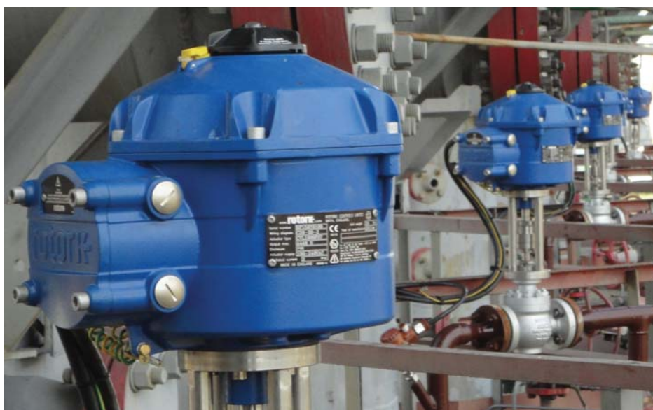
CVA electric control valve actuators recently installed at a Ukrainian compressor station on the pipeline network supplying Western Europe with natural gas from Russia and Central Asia.
